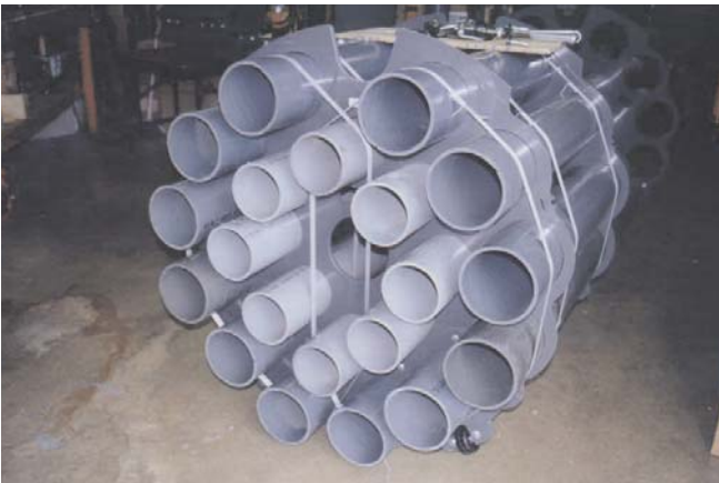
23. Above is a view of a completed bore spacer, conduit and strapping assembly.
